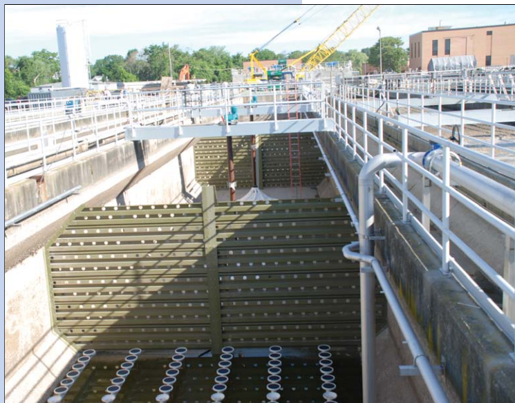
Figure 1. Stratford aeration tank.
